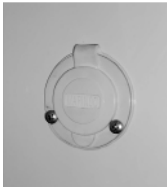
Utility Heat Tape Receptacle
