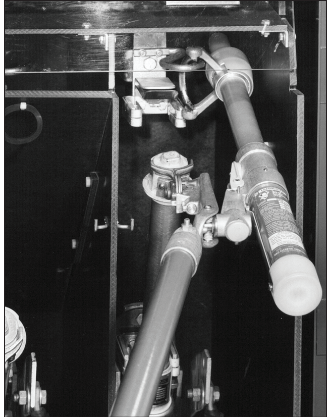
Figure 10. The Loadbuster tool in a Tripped position.
